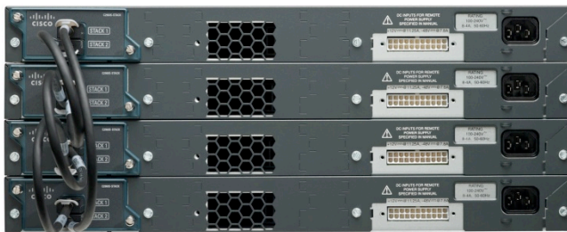
Figure 3. Cisco Catalyst 2960-S Switches with Cisco FlexStack Modules and Stack Cabling
